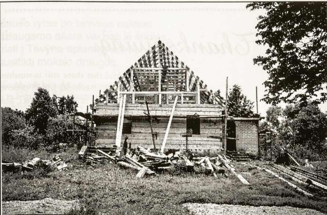
The new house currently being built, but in need of funds for purchase of remaining building supplies.
